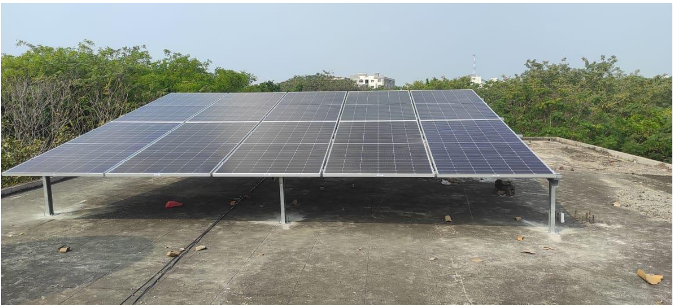
New solar power plant 5 KW capacity installed on roof top of administrative block.
